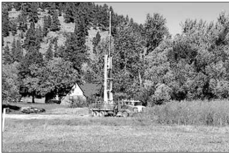
Excel Drilling first tested a well on the Marks property in Clancy in 2024.
